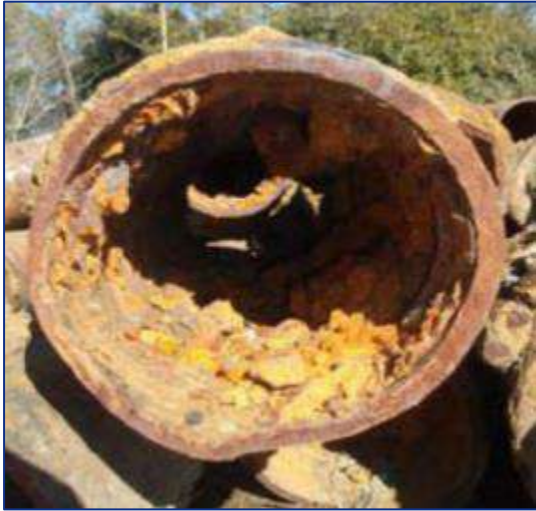
Internal corrosion of cast iron pipe
