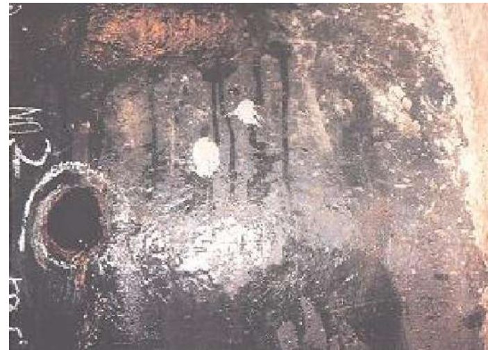
Part corrosion of the steel pipe
