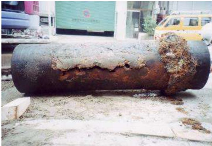
Pipe body corrosion by the corrosive soil
