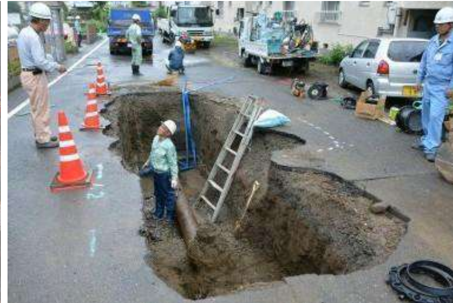
Cave in the road caused by water leakage in Oita City
